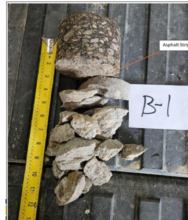
Topeka Blvd. Core Failed Base Concrete Material
