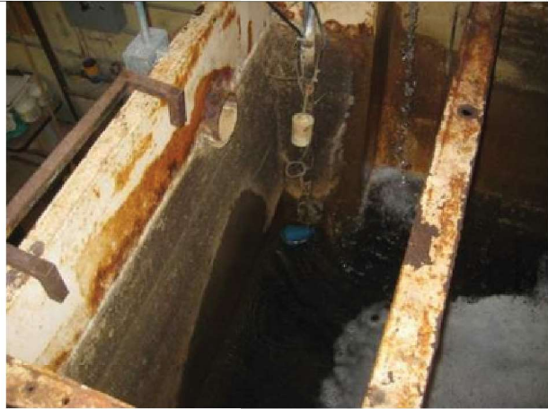
Tank water level controls.
