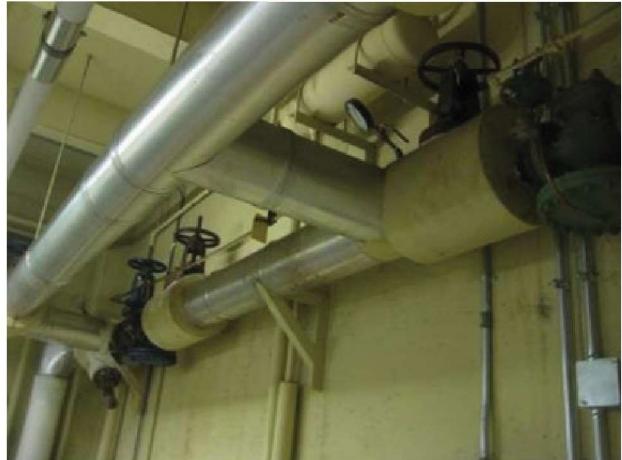
Steam PRV station near tunnel entrance.
