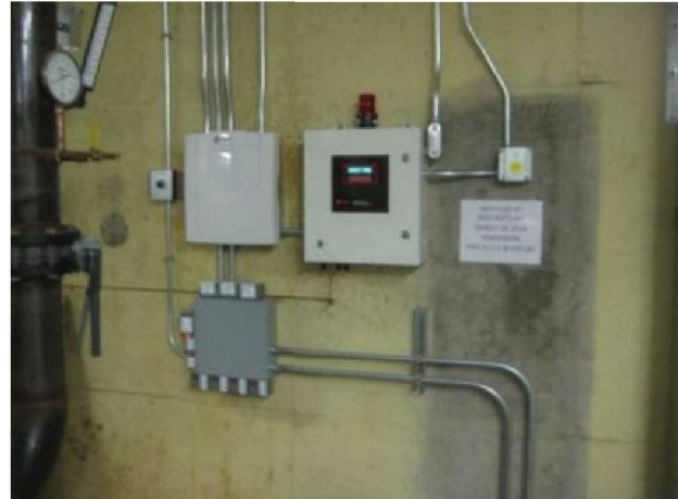
Chiller plant refrigerant monitoring system.
