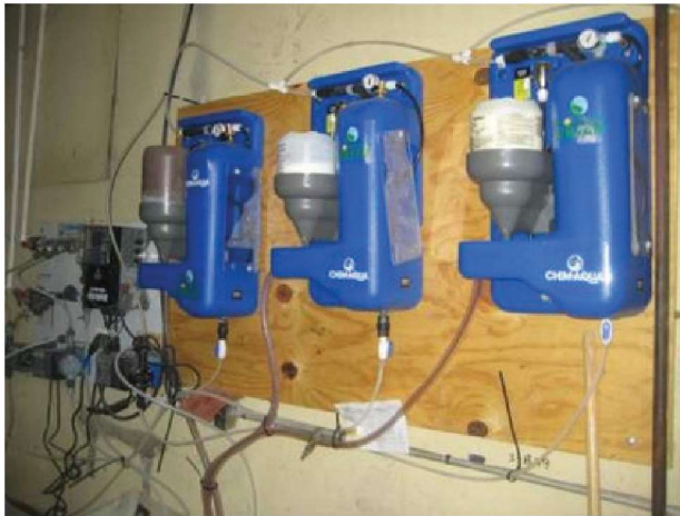
Tower / condenser water chemical treatment.
