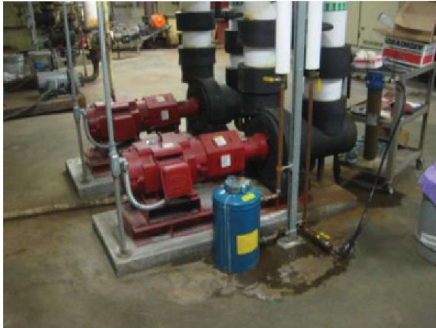
New (2013) chilled water pumps.
