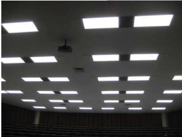
Auditorium Classroom 100 fluorescent fixtures.
