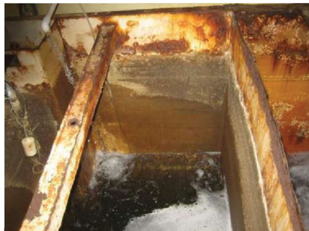
Water level control compartment of tower basin.
