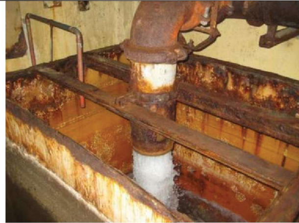
In general tank is very rusted.
