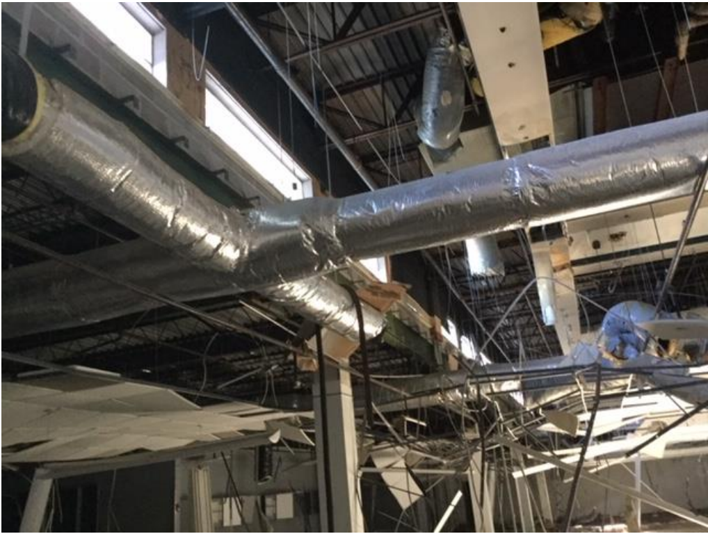
Dismantled ventilation duct, dangling ceiling supports
