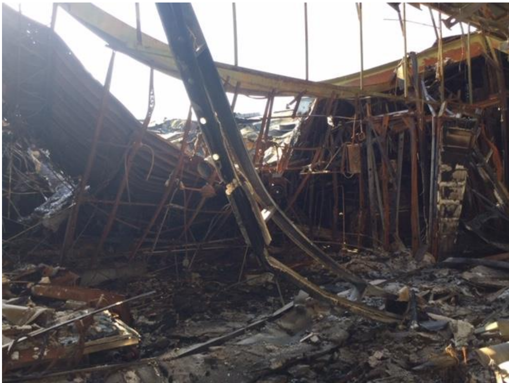
Roof supports collapsed load bearing walls collapsed
