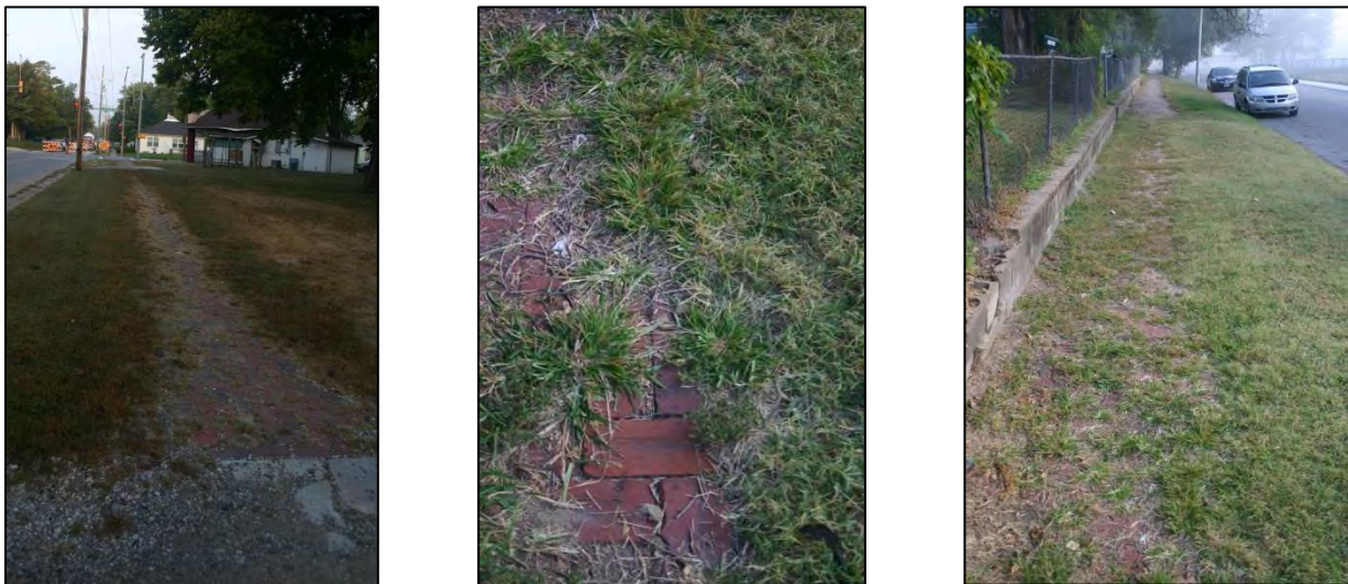
Figure 1: Examples of Sidewalks Needing Repairs Adjacent to Quincy Elementary School
