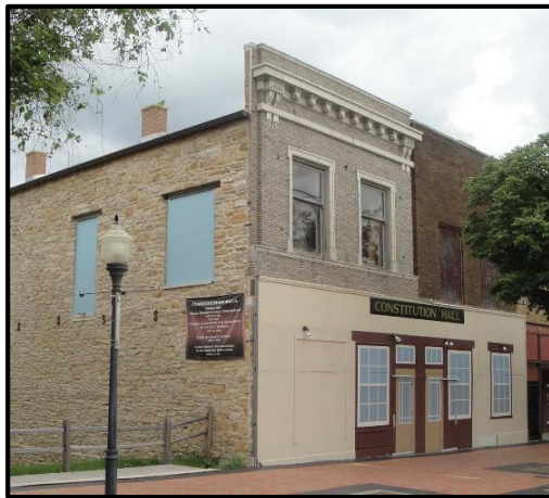
Left, 2015 view of building showing its conglomeration of decayed facades
