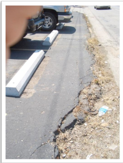
Deteriorating curb and gutter along SW 37th Street west of SW Topeka Boulevard.
