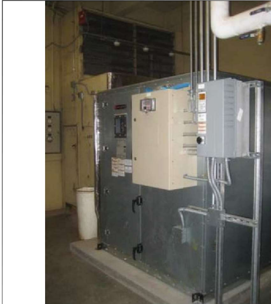
AHU-1 fan has been replaced and VFD provided.
