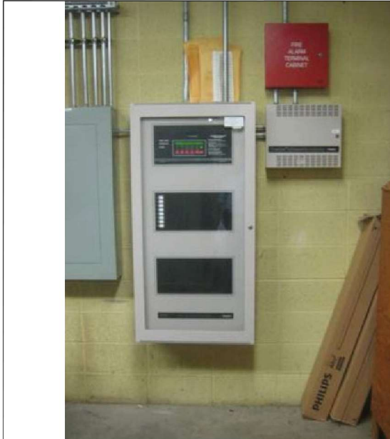
Simplex 4100 addressable main fire alarm control panel. Condition good.
