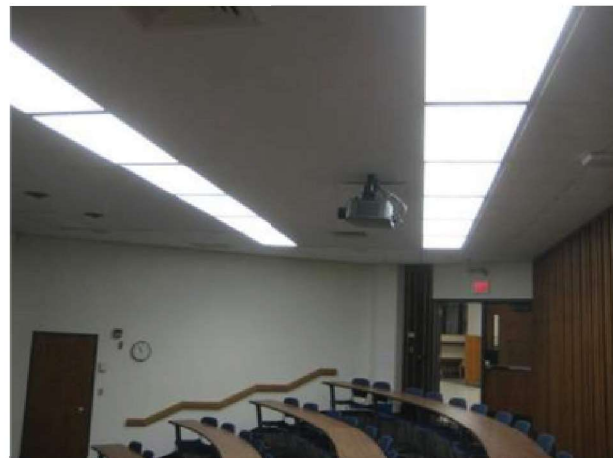
Typical classroom fluorescent troffers are original and have been retrofitted with electronic ballasts and T8 lamps. Similar for all fluorescent lighting throughout building.
