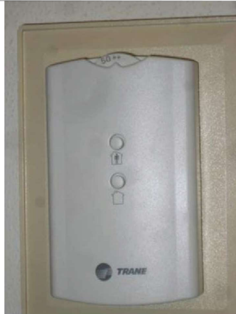
Typical Trane zone thermostat (2013) with OCC/UNOCC push button. Notice setpoint, set at max cooling which may indicate capacity or other system deficiencies or setpoint issues.
