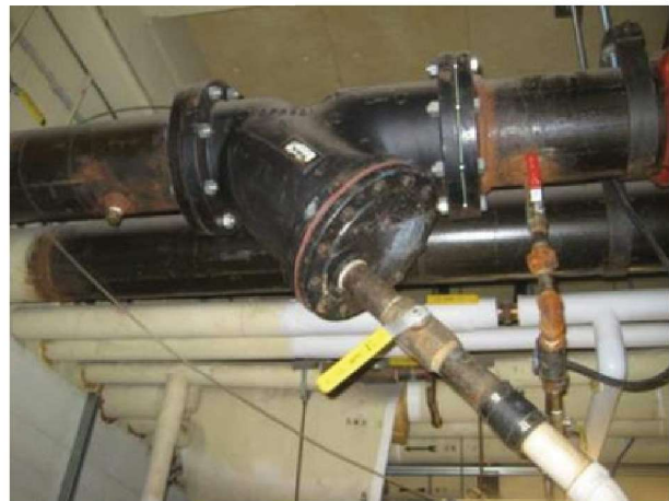
Tower return strainer is leaking, needs repair and new seals. Steel tower piping should be checked for excessive pitting and erosion especially at bottom of vertical drop from penthouse.
