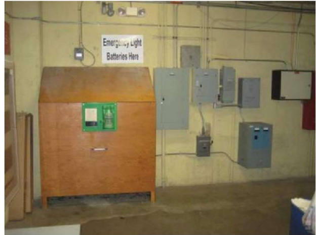
Lead-acid battery system with emergency lighting inverter on wall at right serves all egress lighting in building.
