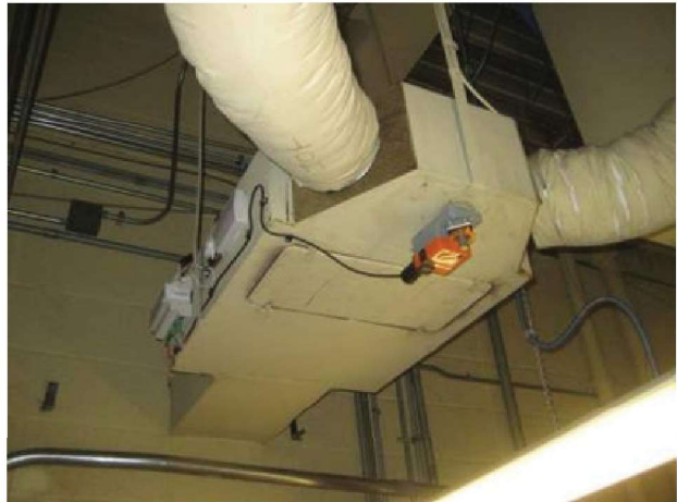
Typical original dual-duct zone box throughout facility with new (2013) Trane control retrofit. Dual duct system and associated boxes are not compliant with modern energy codes as they mix cold and hot energy resources.
