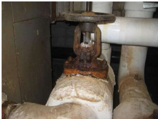
Typical OS&Y gate isolation valves at AHUs are rusted and need replacement with ball valves or butterfly valves.
