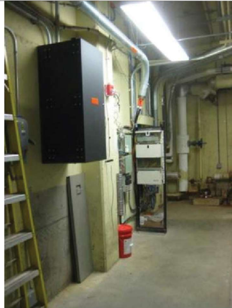
Main building IT and fiber entrance exposed behind substation.
