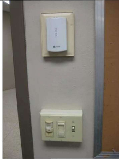
Typical small classroom thermostat and lighting controls with motion sensor retrofit.
