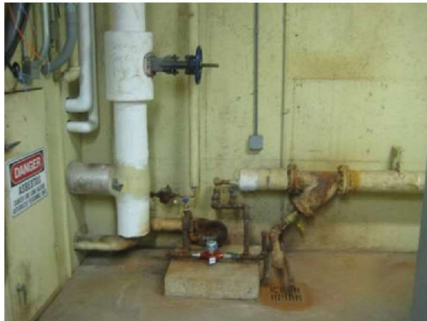
Campus steam supply and condensate return at tunnel. Traps, strainers and valves should be replaced. Long term replacement with gas heating system is recommended.
