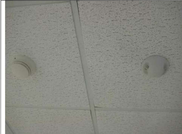
Typical classroom smoke detector and lighting control motion sensor.
