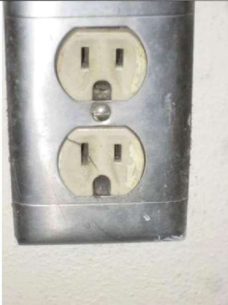
Many original receptacles are cracked and worn, are no longer code compliant.
