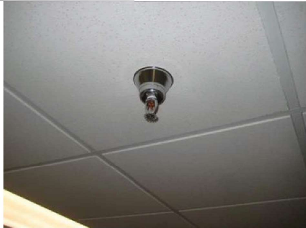
Typical “newer” basement sprinkler head located in past basement renovation areas. Only basement is sprinkled.
