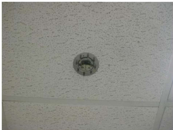
At basement, all original fused link type sprinkler heads need replacement with modern quick-response heads.
