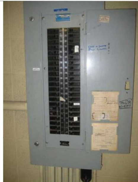
Typical original branch panelboard. Parts no longer made. Panels full. Replacement recommended.
