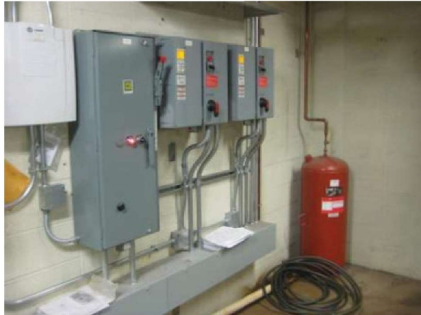
New chilled water plant VFDs and motor starters (2013).
