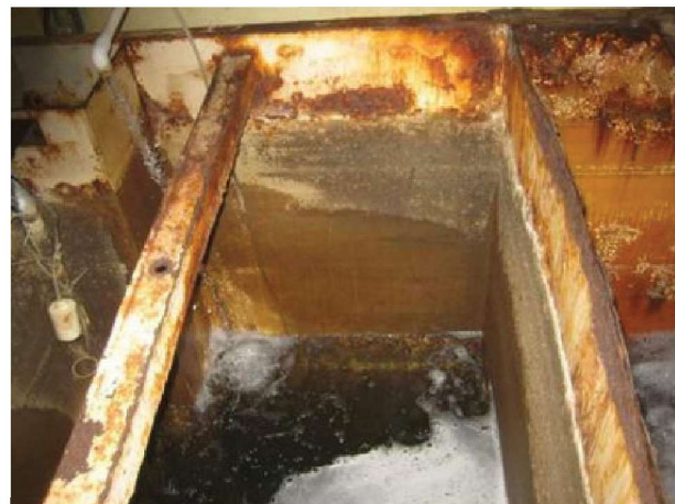
Water level control compartment of tower basin.
