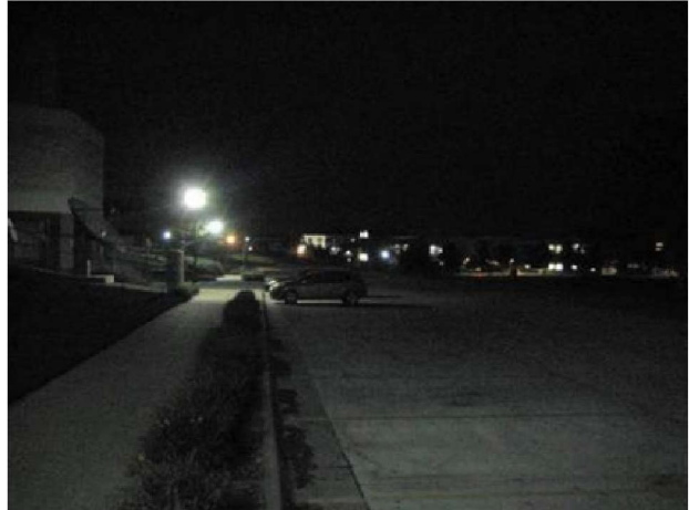
Inadequate lighting at south parking. Appears to utilize inefficient metal halide sources/lamps.
