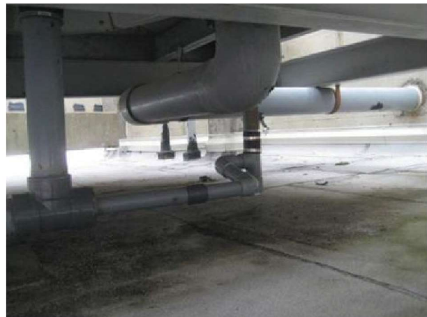
Cooling tower CPVC return piping is in good condition.
