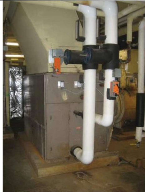
Original built-up single zone AHU-3 similar to AHU-4.
