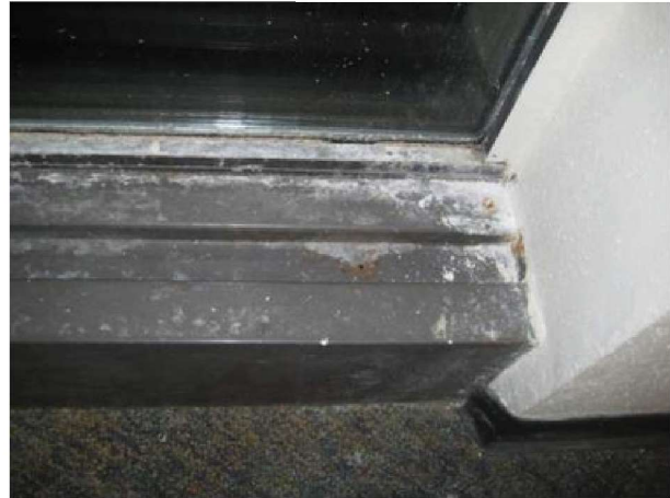
Various window assemblies leak at perimeter and sill.
