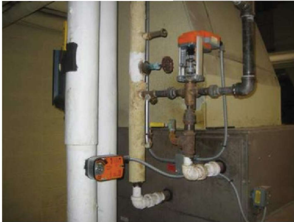
All AHU hot water valves are 3-way with no balancing or flow control valves. 2-way valves with flow control are recommended for energy savings.
