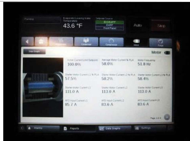
Chiller capacity limit is set at 100%. A lower setpoint should be received/considered for electrical demand savings. Typical capacity during significant load conditions is less than 60% as indicated above (57.5%)
