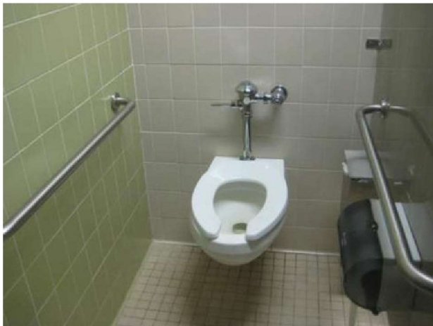
Some accessibility improvements have been implemented throughout facility but typically are not fully compliant with ADA regulations. Significant accessibility improvements are necessary for compliance.
