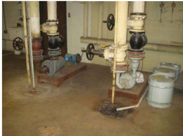
Original constant speed hot water pumps, valves and pads need replacement. Pumps lack suction diffusers, strainers and balancing valves. New pumps, accessories and VFD operation is recommended.
