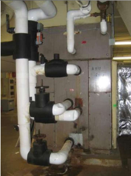
Original dual-duct AHU-2 CW/HW coil section. Needs replacement.
