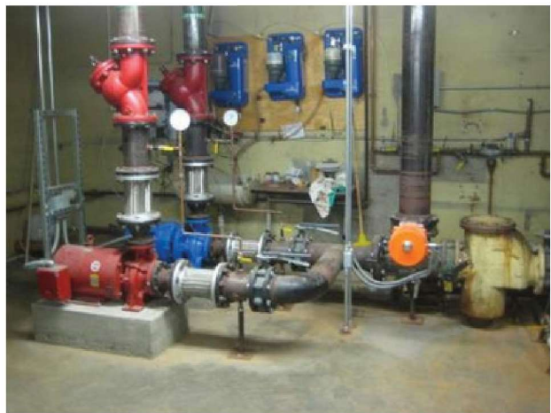
Cooling tower / condenser water pumps. Single basket strainer requires system shutdown to clean. Lack of automatic filtration system requires regular manual cleaning and flushing of strainers.
