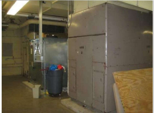
Original dual-duct AHU-2. Fan section replaced in 2013 .
