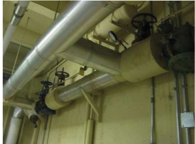
Steam PRV station near tunnel entrance.
