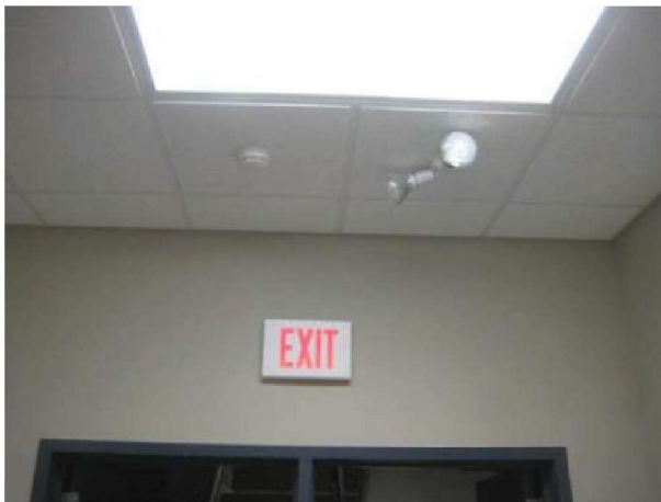
Typical surface emergency lighting screw-in lamp holder/fixture. Overall emergency lighting coverage is fair. A mock power outage is recommended to determine actual performance and identify areas needing improvement.
