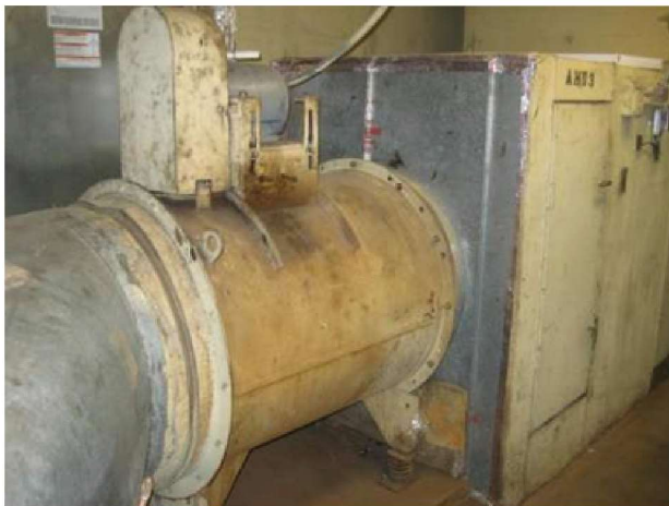
Original AHU-3 axial flow fan.
