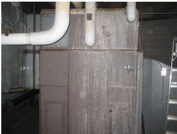
Original dual-duct AHU-6 in penthouse mechanical room. Note history of condensation at casing. Needs replacement.
