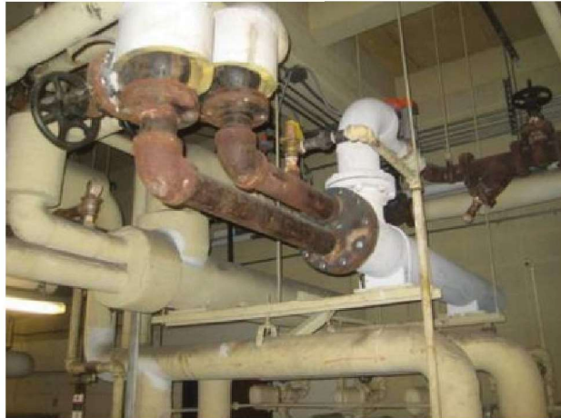
Original heating plant steam HW converters. Overall steam-to-HW process is a very inefficient heating method compared to local natural gas boilers.
