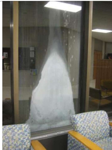
Some window sections have failed with past condensation evident between panes.
