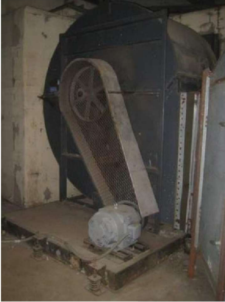
Original AHU-6 supply fan needs replacement. Inlet vanes have been disconnected and new VFD provides air modulation.
