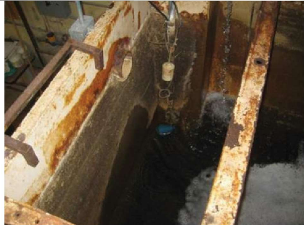
Tank water level controls.
