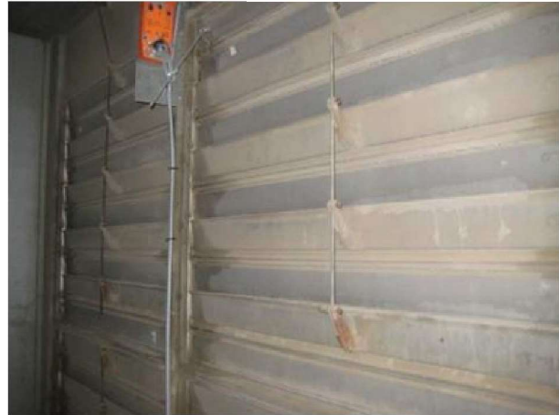
AHU-6 outside air dampers with replacement actuators.
