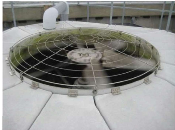
Cooling tower fan has gear box vibration. Needs investigation.
