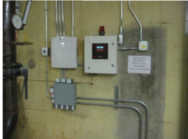
Chiller plant refrigerant monitoring system.
