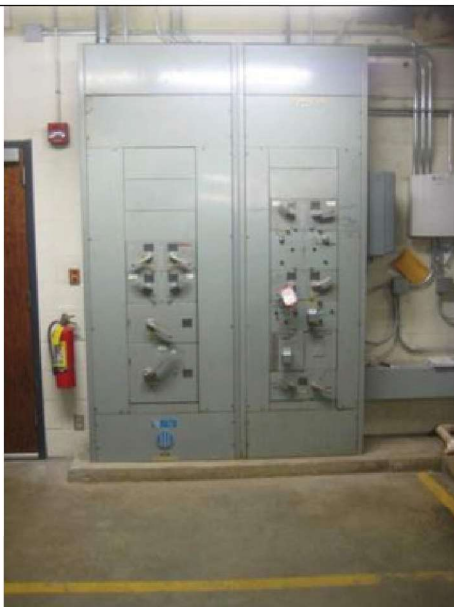
Motor control center needs replacement.
