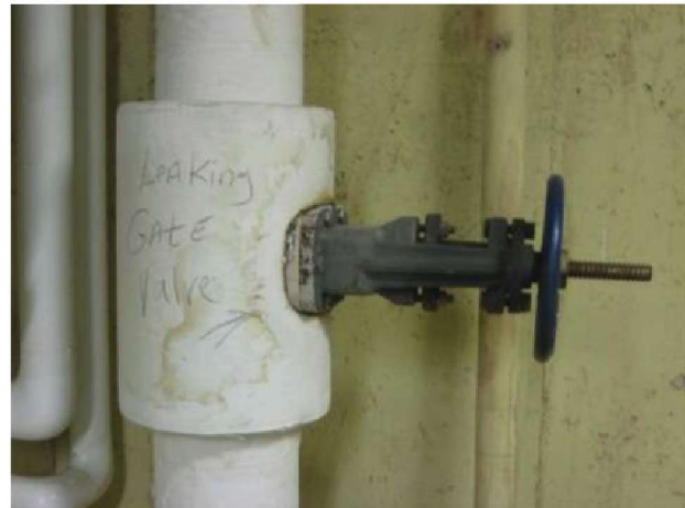
Main steam shut-off valve indicated to leak. Leaking steam a safety hazard due to high pressure/temperature steam.
