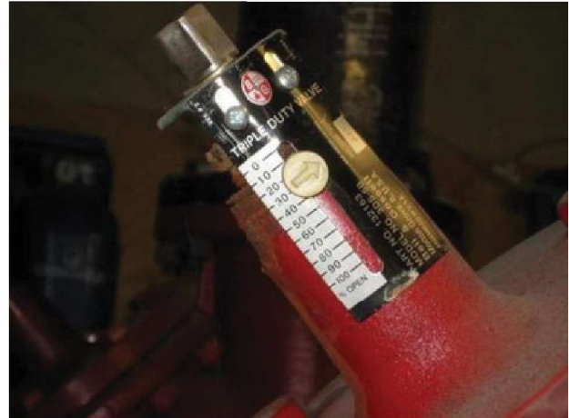
Cooling tower pump 3D valves are 72% restricted to limit flow. Very wasteful parasitic energy loss. VFDs recommended.
