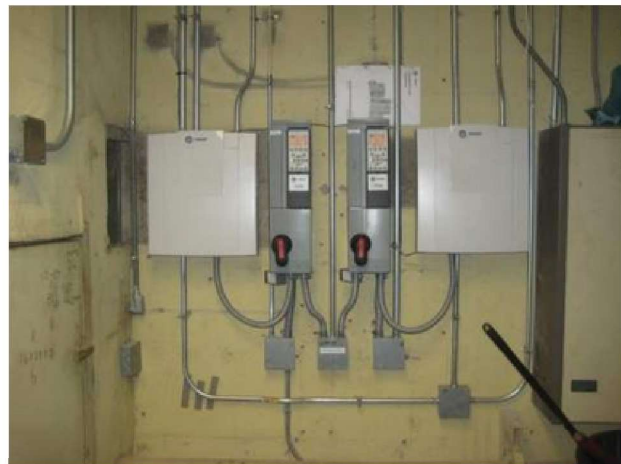
New AHU-3 and AHU-4 VFDs. At fans original inlet vanes are in fixed position.
