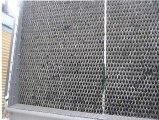
Cooling tower fill needs replacement. Chemical treatment needs adjustment to lessen scale.
