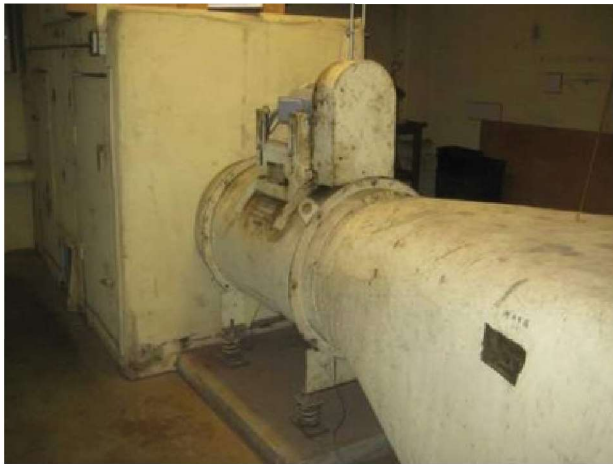
AHU-4 fan and mixing box need replacement.
