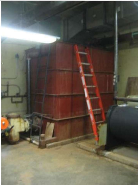
Original remote cooling tower basin is rusted and needs replacement. Removal and use of tower sump is recommended.
