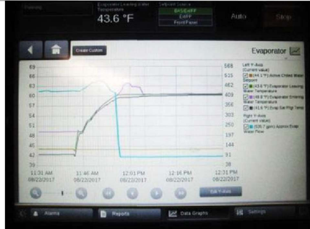
Chiller shut down during occupied time 11:40am (Tuesday 8/22) during significant load conditions. Reason unknown. History should be reviewed.
