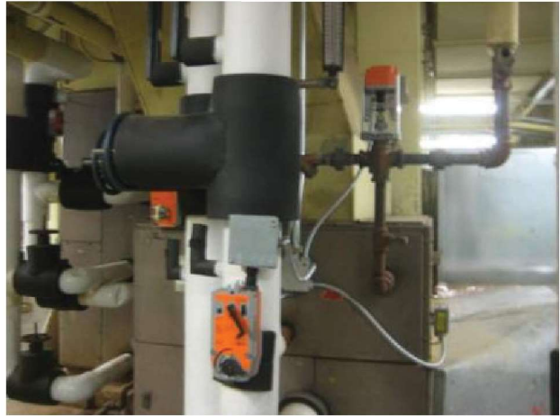
AHU-3 (shown) and all AHUs lack CW and HW flow limiting valves which lessens energy savings possible with variable speed pumping (CW only).
