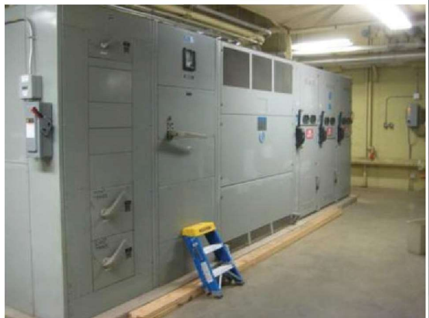
Original main electrical service: 1600A, 1000 KVA substation fed from campus 4160 volt west primary loop. Transformer efficiency is poor compared to modern equipment. Original manufacturer is defunct and switchgear parts are not available. Replacement with modern circuit breaker substation is recommended. MV switches at end will require replacement if campus voltage increased.
