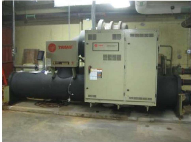
New (2013) 280 ton centrifugal chiller with VSD capacity modulation.
