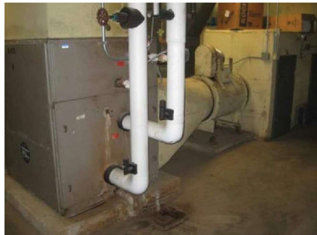
Original built-up AHU-4. Single zone with hot/cold deck mixing. Overall condition poor to fair.
