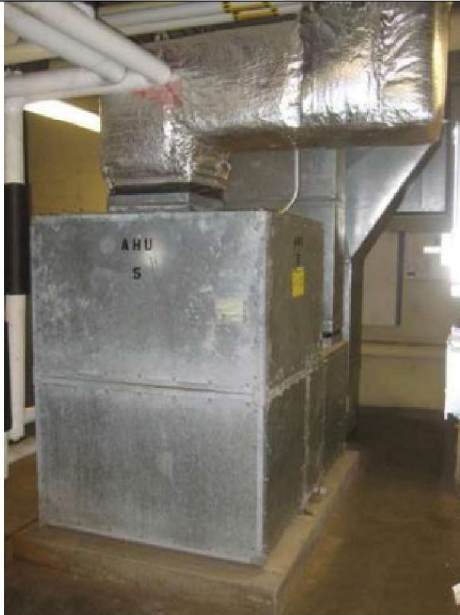
Cooling-only VAV AHU-5. Original dual deck unit replaced to serve VAV box zones.
