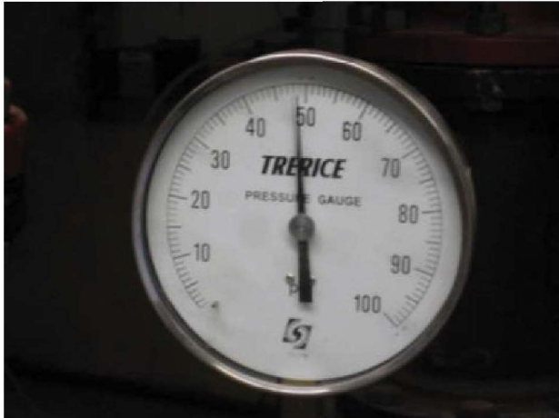
Cooling tower pump pressure gauge (upstream of 30 valve) 49 PSI of pump pressure is required to pump from basement to rooftop tower. Very energy intensive. Redundant pumps are 30 HP each.
