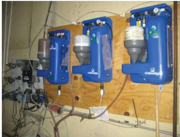
Tower / condenser water chemical treatment.
