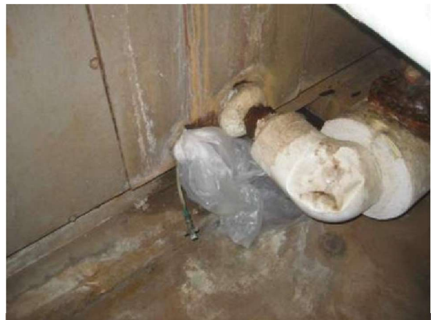
Drain pan at AHU-6 is rusted and leaking at penthouse.
