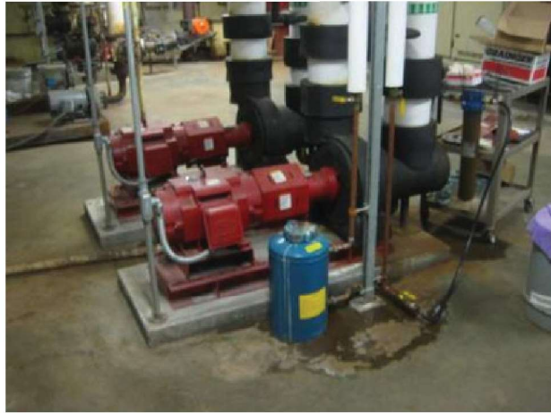
New (2013) chilled water pumps.
