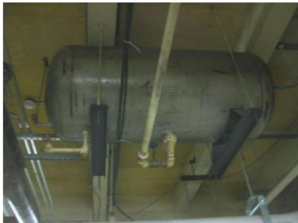
Original HW system expansion tank at structure needs replacement. Old technology tank lacks bladder for air separation and pressure control. New tank would be at floor for ready inspection and maintenance.
