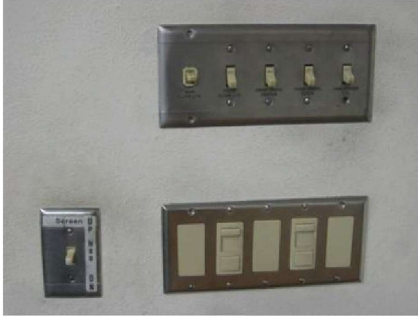
Typical large classroom lighting controls are mostly original. Dimmers are not suitable for fluorescent lamp dimming.
