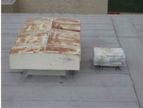
Rooftop intake and relief penthouses are dented and rusted, need replacement.
