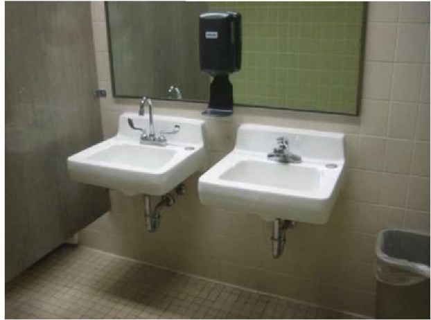
Typical manual faucet controls, trap guards missing.
