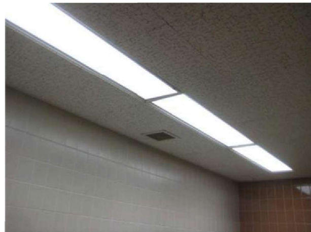
Typical small exhaust grille at restrooms. Restroom exhaust in general is inadequate.
