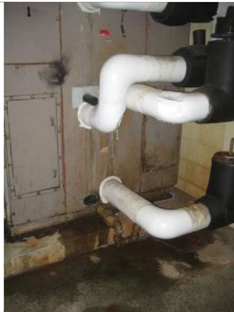
Original dual-duct AHU-1. Drain pan is leaking and casing is rusting.
