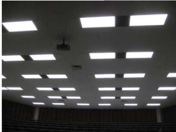
Auditorium Classroom 100 fluorescent fixtures.
