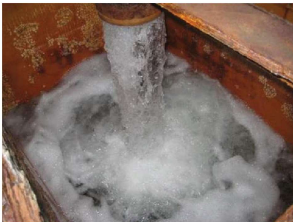
Receiving / surge compartment of remote tower basin.
