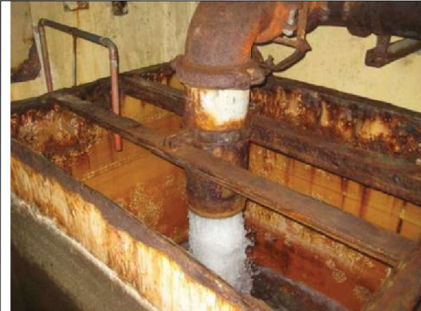
In general tank is very rusted.
