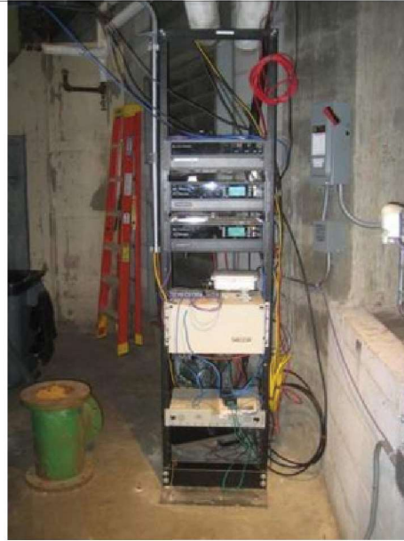
KTWU transmitter rack is located exposed in penthouse mechanical room. Additional protection is recommended.
