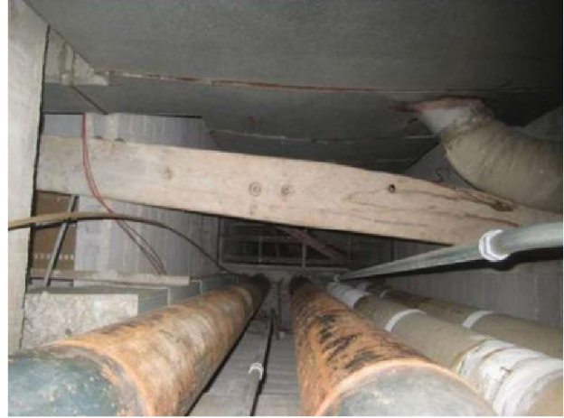
South AHU-6 return air shaft is open to all floor return air plenums. Also shares chilled and condenser water piping. No longer meets codes for fire and smoke containment.
