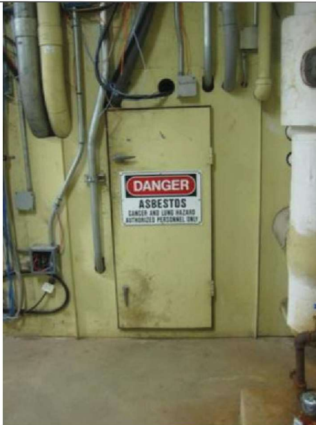
Asbestos indicated at tunnel systems. Appears most building piping systems have been abated.
